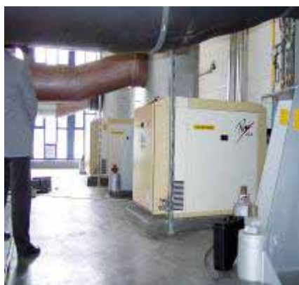
Figure 42: CHP-units in the boiler house
