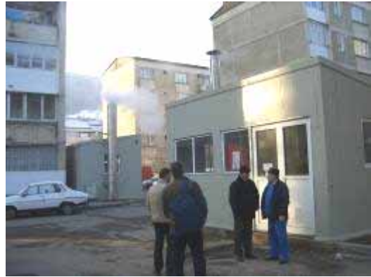
Figure 32: Modernised block boiler units in a standardised container construction
