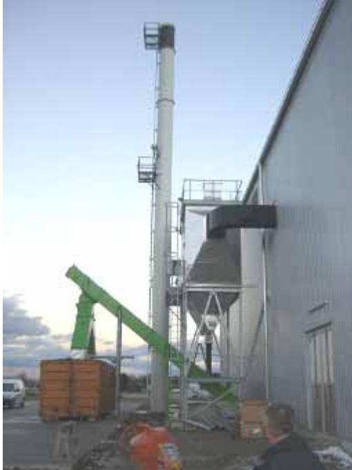
Figure 7: Biomass CHP Ternitz
