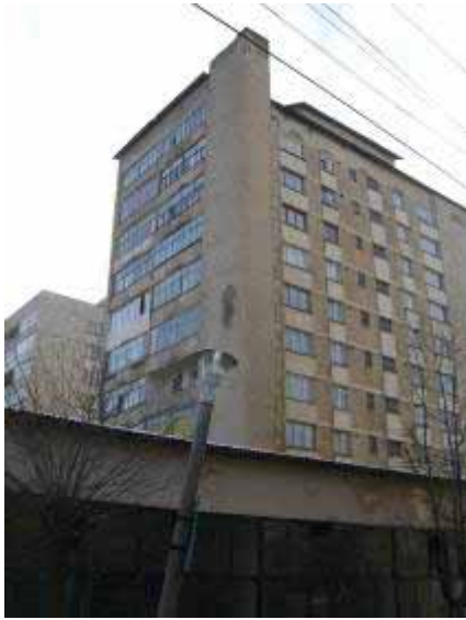
Figure 31: Block boiler unit, the funnel is attached to the residential building
