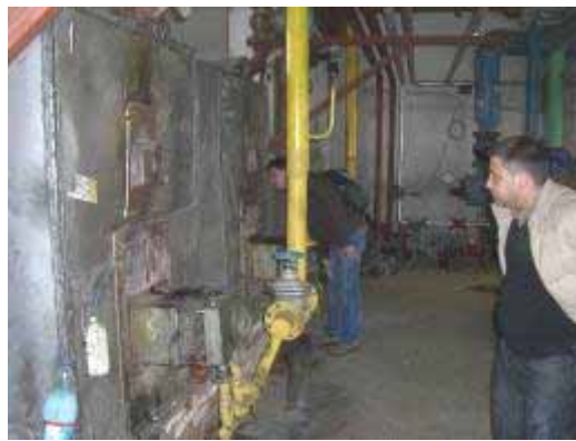
Figure 30: Old gas boilers – 500 kW
