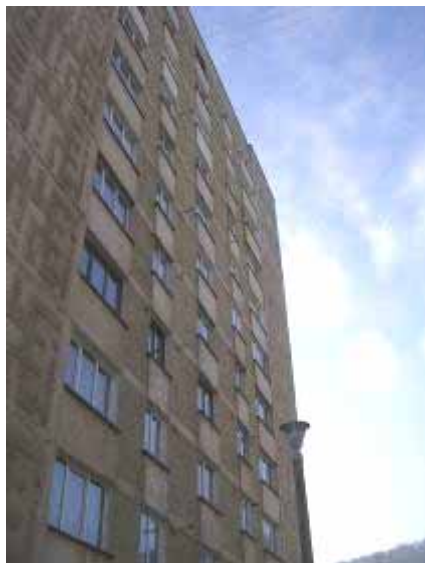
Figure 35: DH supplied building with numerous flats, which have switched to individual gasetagenheizungen – see the funnel next to the windows
