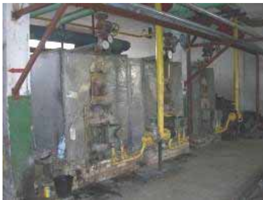
Figure 29: Old gas boilers – 500 kW, the burner can only be regulated manually
