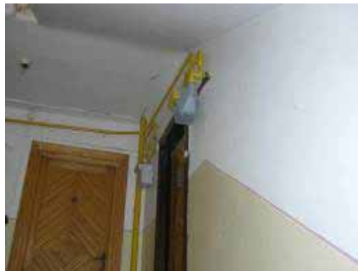
Figure 36: Individual gas supply in flats in a DH supplied building
