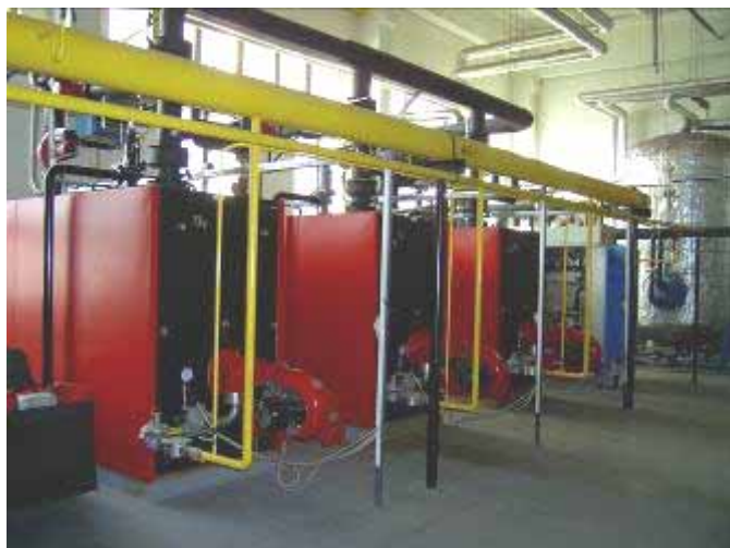
Figure 38: The natural gas fired boilers
