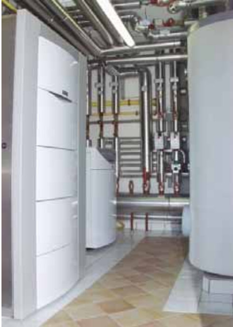
Figure 5 Vaillant's 4,5 kW el PEFC residential fuel cell system installed in Hotel Ochensberger (Source: Vaillant Vienna)
